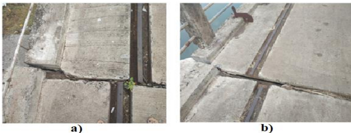
Figure 2. a) Displaced deck slab; b) Damaged expansion joint.
