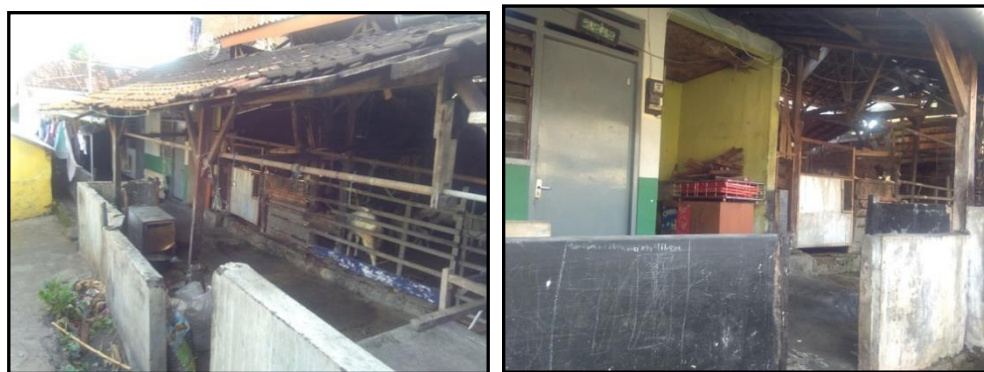
Figure 4. Interior Condition of Ahmad's House, 2019. Source: Researcher Documentation
