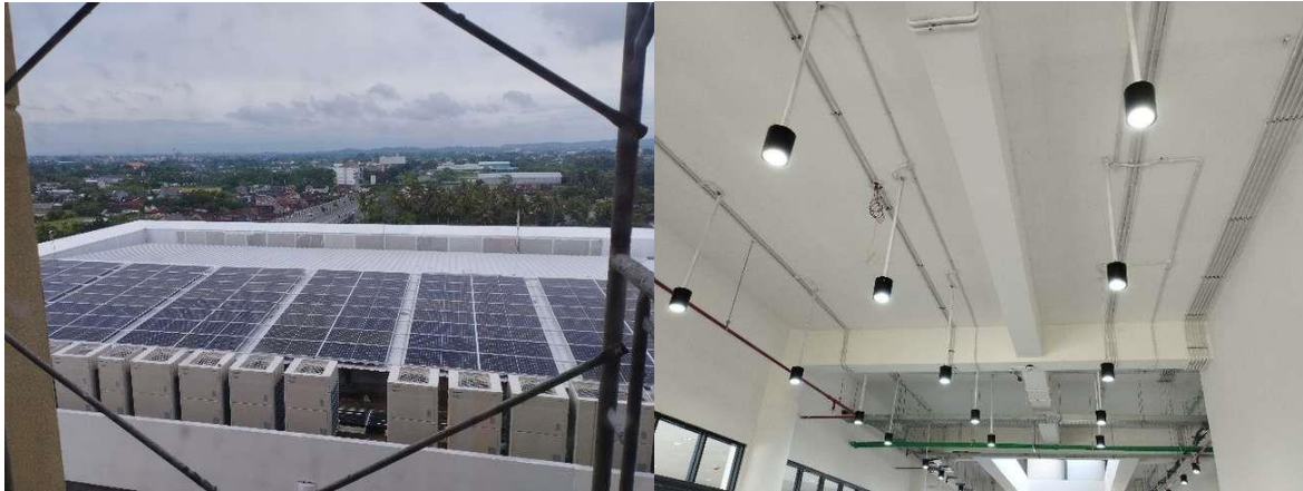
Figure 8: a) Photovoltaic in UNU Yogyakarta Campus Building, b) Lighting Source: author, 2023
