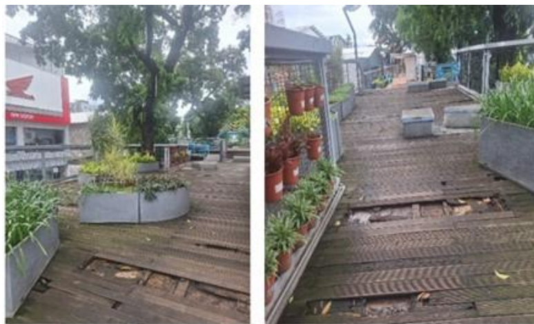
Figure 3. Poorly maintained park conditions, 2025. (Source: Personal)
