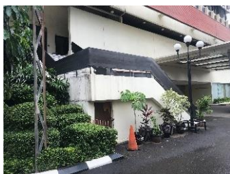
a. The access to the building was only a staircase without a ramp
