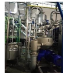
d. Oil tank
