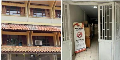
Figure 2. Building age damage
