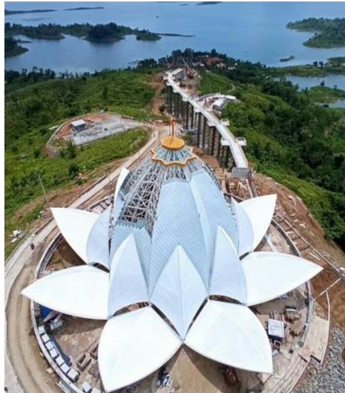
Figure 2. Progress of construction of the Al-Kamil Mosque Source: PT Indi Daya Karya Contractor Documentation for 2021
