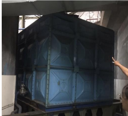
Figure 8. Majesty Apartment Rooftop Tank Source: Private Assets
