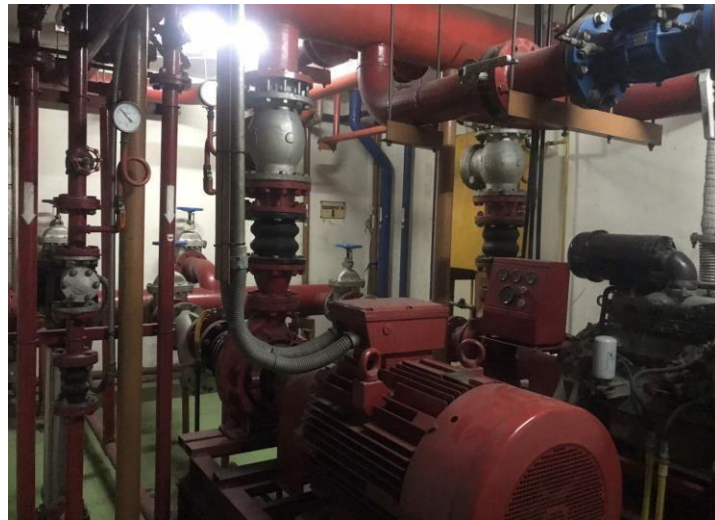
Figure 14. Hydrant Room at Majesty Apartemen Source: Private Assets
