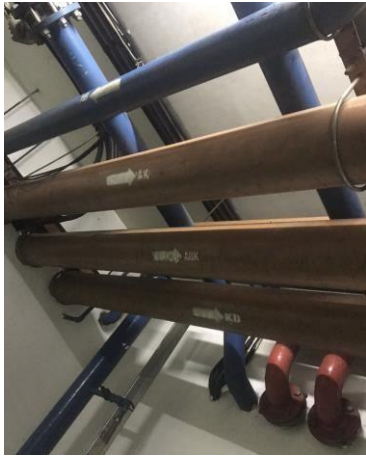
Figure 11. Majesty Apartment Dirty Water Pipe
