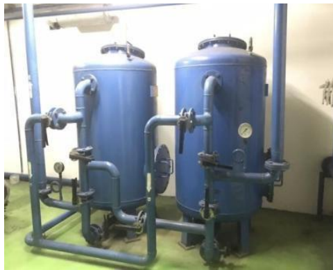
Figure 4. Clean Water Tank Majesty Apartment Source: Private Assets
