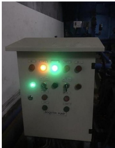
Figure 7. Majesty Apartment Booster Pump Panel Source: Private Assets
