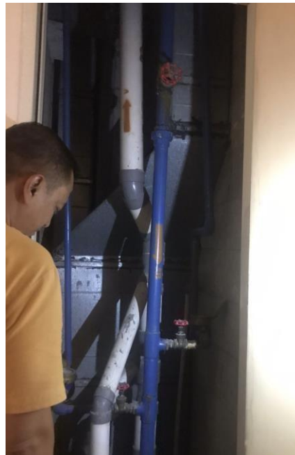
Figure 10. Main pipe next to the bathroom of Majesty Apartment unit Source: Private Assets
