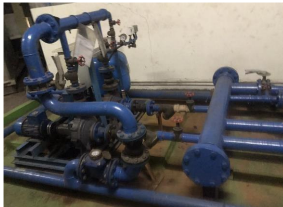
Figure 6. Majesty Apartment Booster Pump Pipe Source: Private Assets
