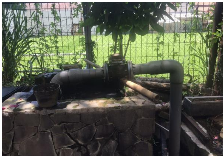
Figure 13. The last tank of dirty water in Majesty Apartment
