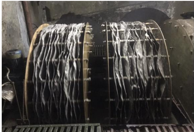
Figure 12. Wastewater Treatment With Fat Trapping in Majesty Apartment
