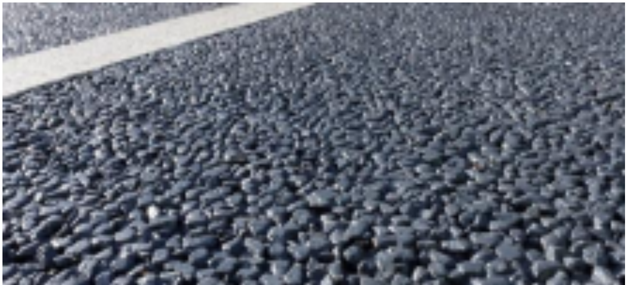
Figure 3. Asphalt with infiltration
