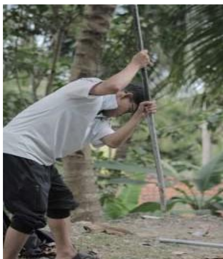
Figure 1. The process of digging a hole for a convex mirror pole Source: Author Documentation 2023
