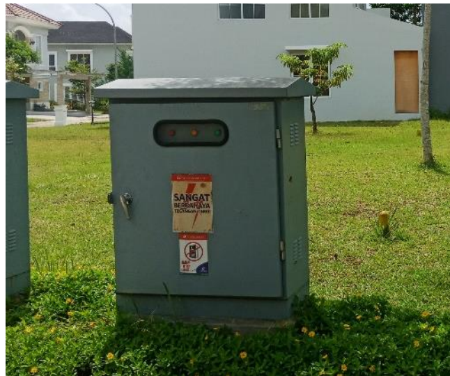
Gambar 10. Electric panel di cluster Sumber: Pribadi
