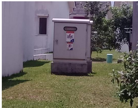
Gambar 3. Electric panel di cluster Sumber: Pribadi
