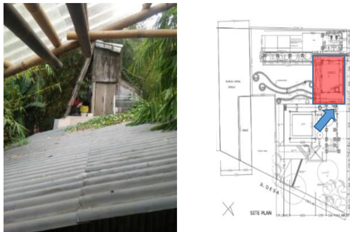
Gambar 3 Material Atap Asbes & Fiberglass Studio Akanoma (Sumber: Data Studio Akanoma & Data Pribadi)
