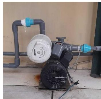
Gambar 17. Jet Pump di Kosan Maysa Raiya No. 87
