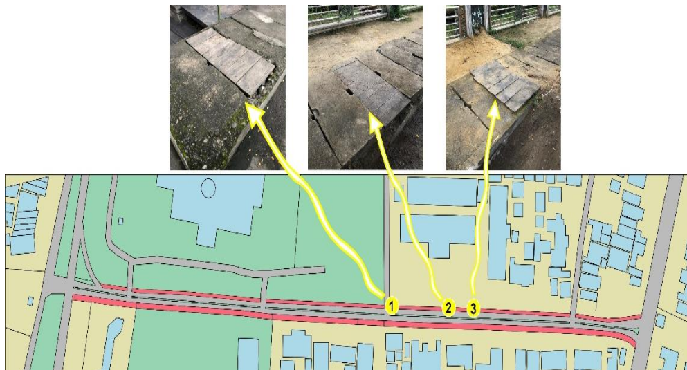
Figure 7. Damage Point on the Left Lane (Source: Author Data, 2024)
