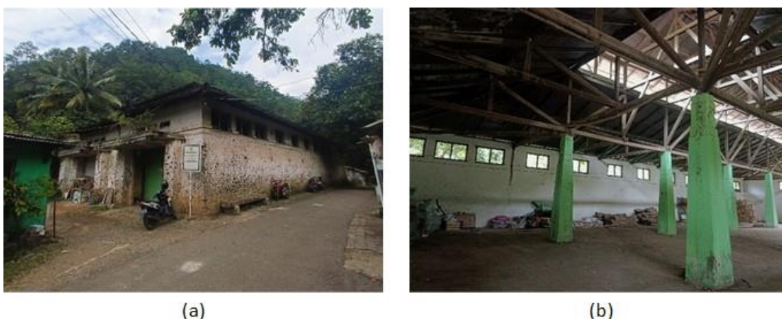
Figure 2. (a) Cililin Radio Station transmitter building (b) Interior and wooden construction of the radio transmitter building.
