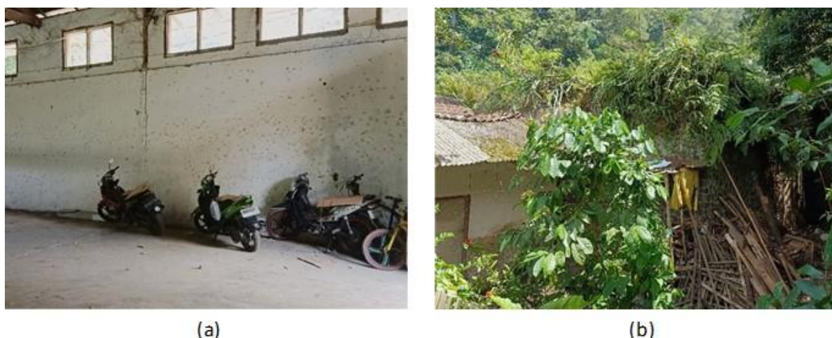
Figure 3. (a) Interior of the building used as a warehouse and vehicle garage (b) Physical degradation of the transformer building.
