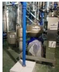
c. Separator tank
